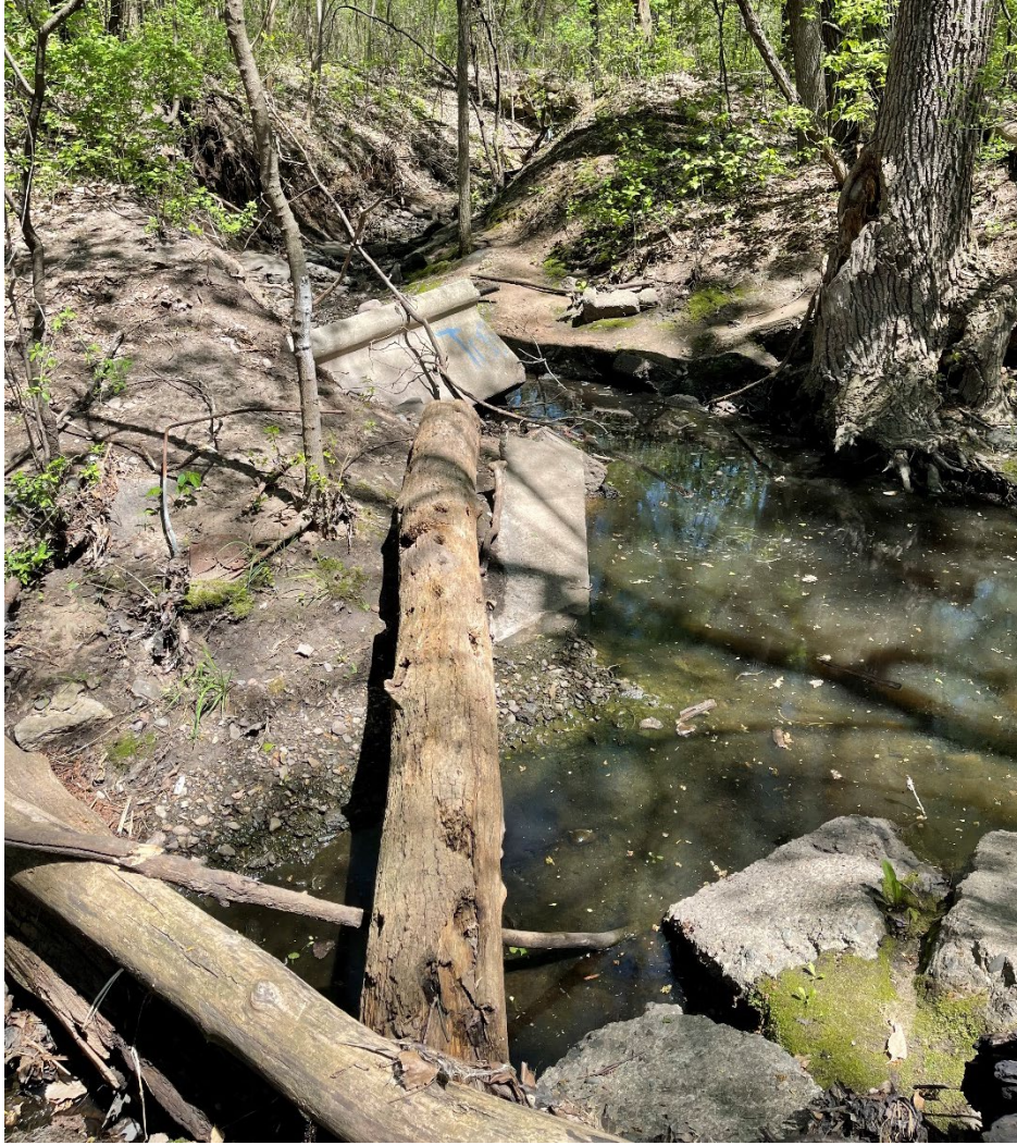
Figure 6-2 Basin J Downstream Outlet Channel Erosion and Construction Debris
